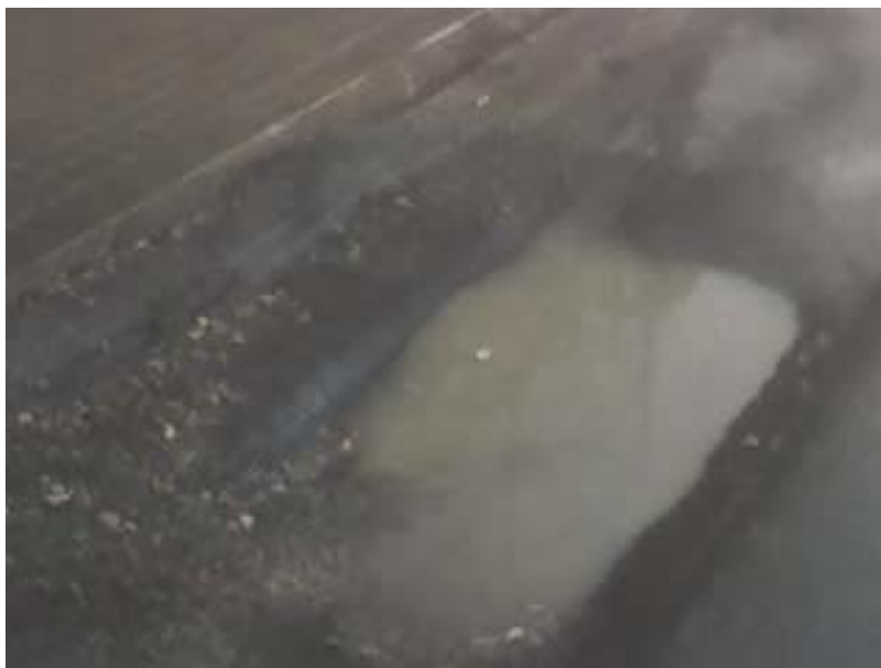
Size and depth of damage to the road.
