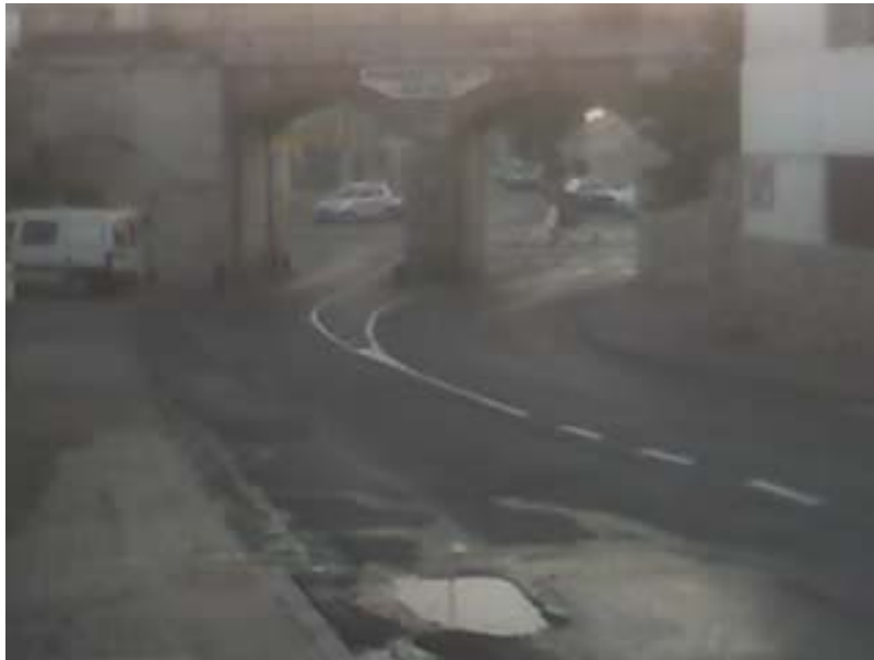
Collapse of road near Ragged Staff Gates last week.
